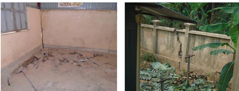
Figure 6. Damages at the primary school (L5 in Figure 3): In the classroom (left) and on the surrounding walls (right).
